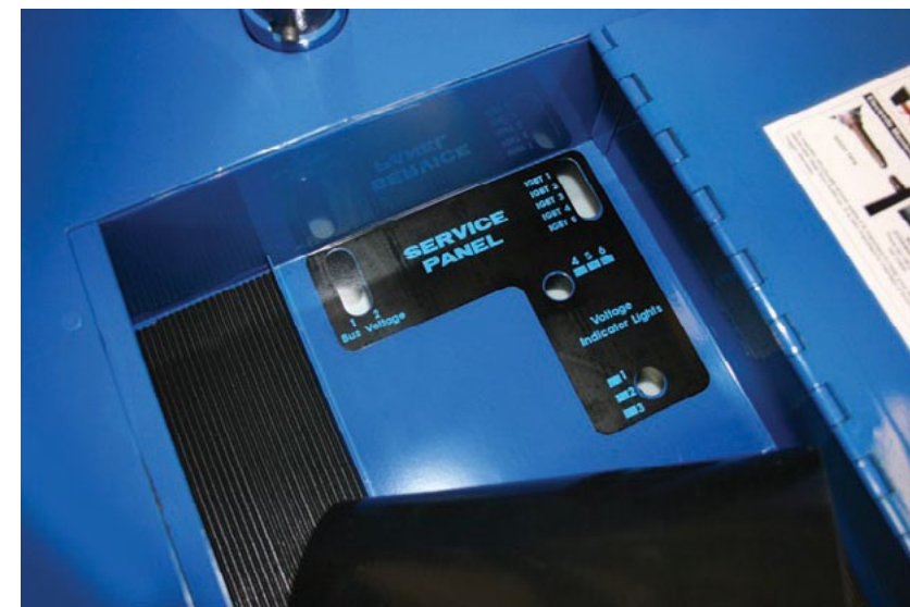
Service Panel Window – Control System Status Lamps
